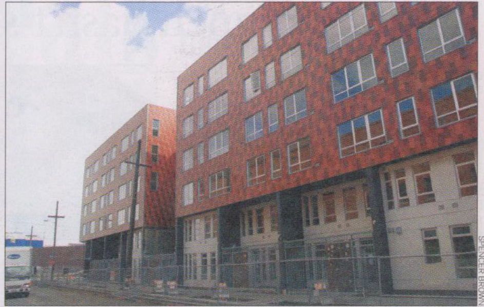
Baker's design for housing is under construction at 888 Seventh St., in San Francisco.
